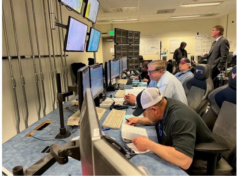
IWTU employees monitor start-up operations from the facility control room.
