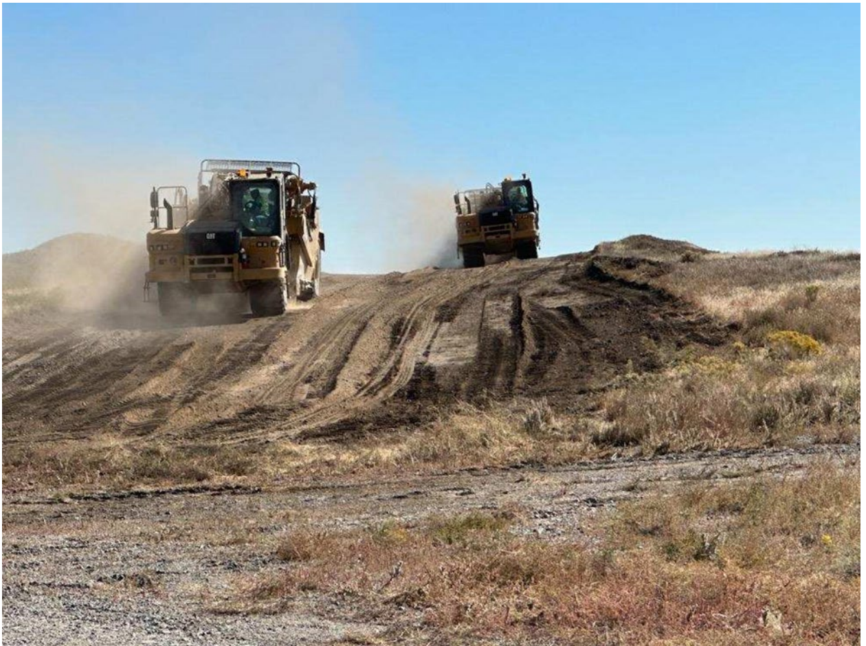
Crews recently broke ground on a new cell for the Idaho Comprehensive Environmental Response, Compensation and Liability Act Disposal Facility, Environmental Management's onsite, engineered landfill for cleanup program waste.
