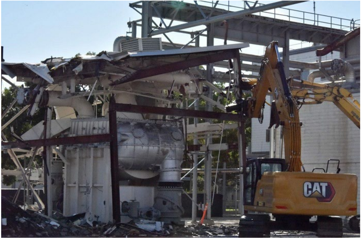
Crews demolish one of two massive steam condensers at the Naval Reactors Facility's Aircraft Carrier 1st Gen. Westinghouse prototype facility. It was the prototype for the USS Enterprise, the nation's first nuclear-powered aircraft carrier.
